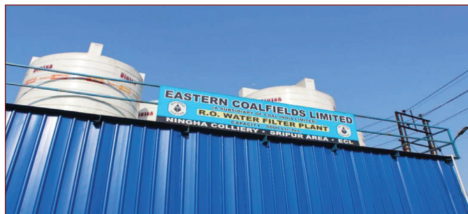
Mine Water Treatment Plant at ECL
